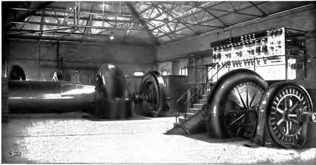
CENTRIFUGAL LIFT PUMPS IN SEWAGE DISPOSAL PLANT—DRIVEN BY SYNCHRONOUS MOTORS DIRECT-CONNECTED—ST. BENARD STATION, NO. 3, NEW ORLEANS, LA.
