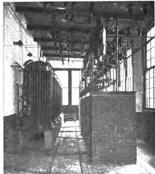
Fig. 6 HIGH TENSION COMPARTMENT, ARDMORE SUBSTATION
