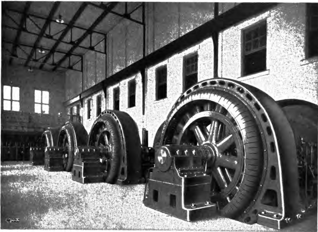
FOUR ATB 2250 KW., 13,200 VOLT, 210 R.P.M. WATERWHEEL-DRIVEN ALTERNATORS ST. ANTHONY FALLS (MINN.) POWER COMPANY
