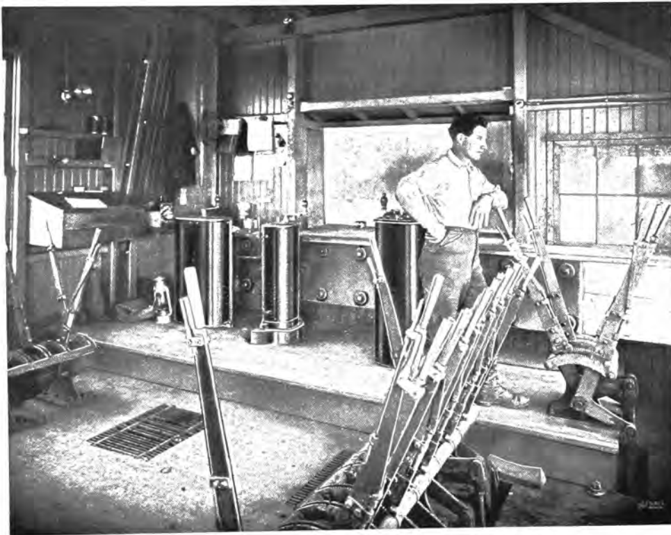
VIEW IN WINCH ROOM OF GOLD DREDGE NATOMA NO. 1 SHOWING CONTROLLERS FOR OPERATING BUCKET LINE, SCREEN AND WINCH MOTORS
