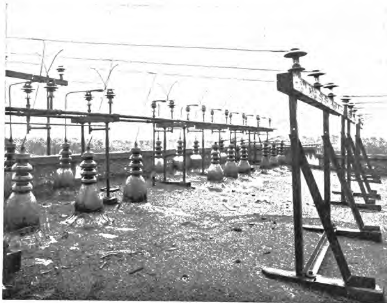
Fig. 12 HIGH TENSION WIRING ON ROOF OF NAVAL ACADEMY SUBSTATION
