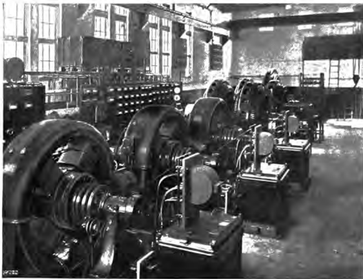
Fig. 6 INTERIOR OF WATERTOWN SUBSTATION
