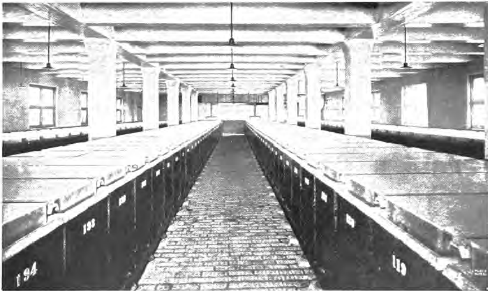
Fig. 30 LOWER BATTERY ROOM
