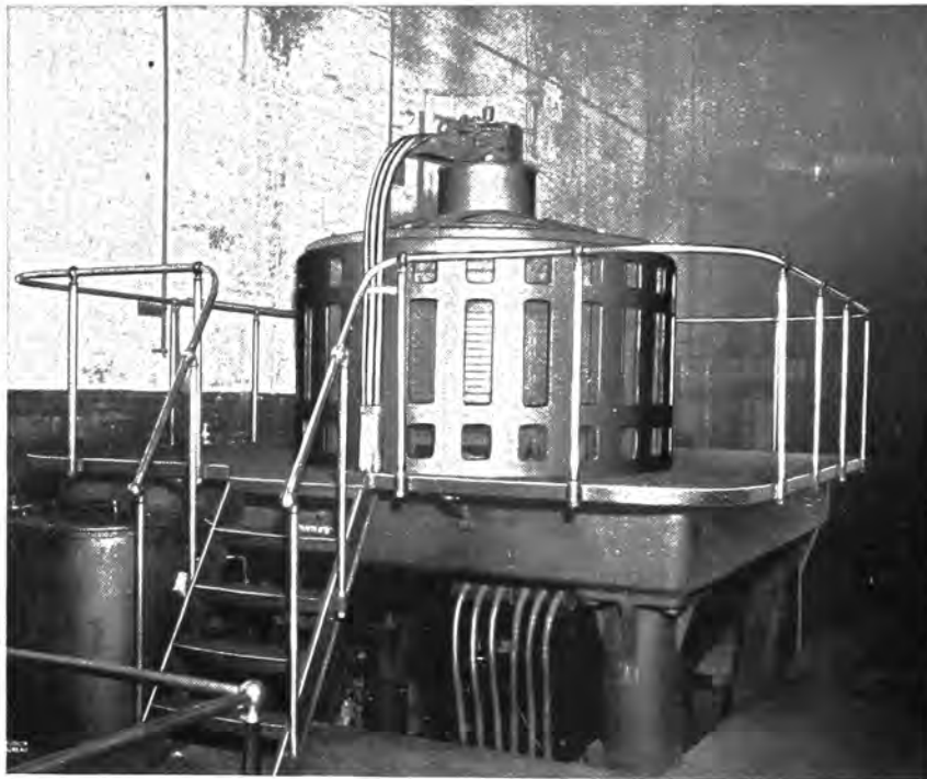
1500 H.P. INDUCTION MOTOR DRIVING CENTRIFUGAL PUMP MUNICIPAL PUMPING PLANT, BUFFALO, N. Y.
