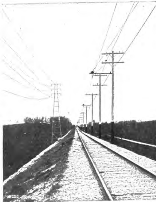
Fig. 16 STANDARD HIGH TENSION TOWER USED ON PRIVATE RIGHT-OF-WAY
