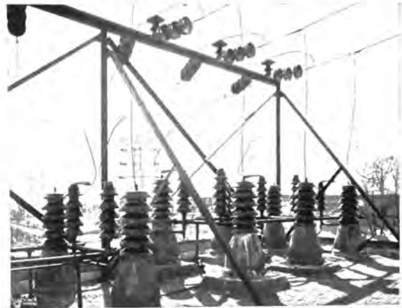
Fig. 20 HIGH TENSION ROOF BUSHINGS
