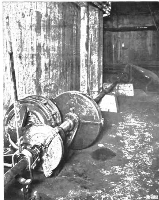
BACK GEARED INDUCTION MOTOR DRIVING TWO CONVEYOR BELTS
