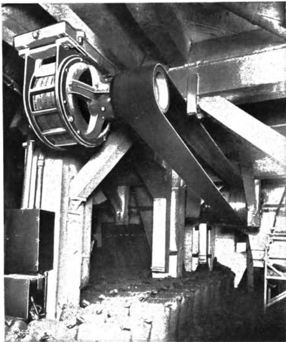
75 H.P. INDUCTION MOTOR SUSPENDED FROM CEILING DRIVING ELEVATORS, MILLS AND CLEANERS. ADY AND CROWE MERCANTILE COMPANY
