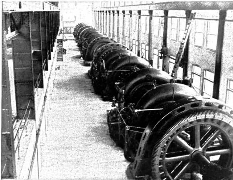
GENERATOR ROOM IN RAINBOW STATION, SHOWING SIX 6000 H.P. GENERATING UNITS
